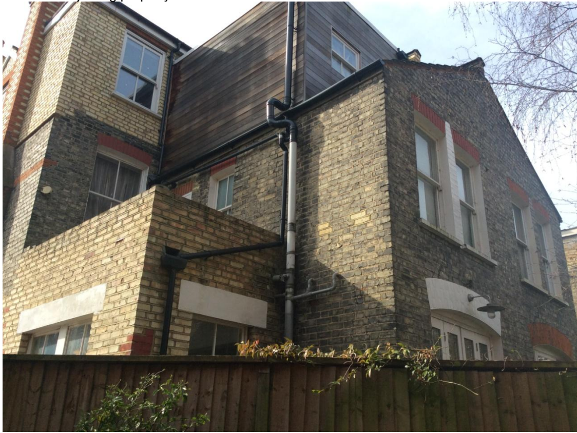
Photos of adjoining property at No. 2 Gisburn Road
